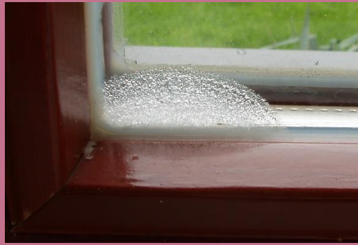
Picture 6.2 – Water attack defect
