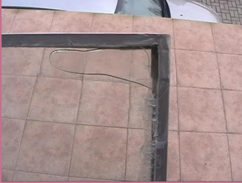
Picture 6.1 – Water attack defect
